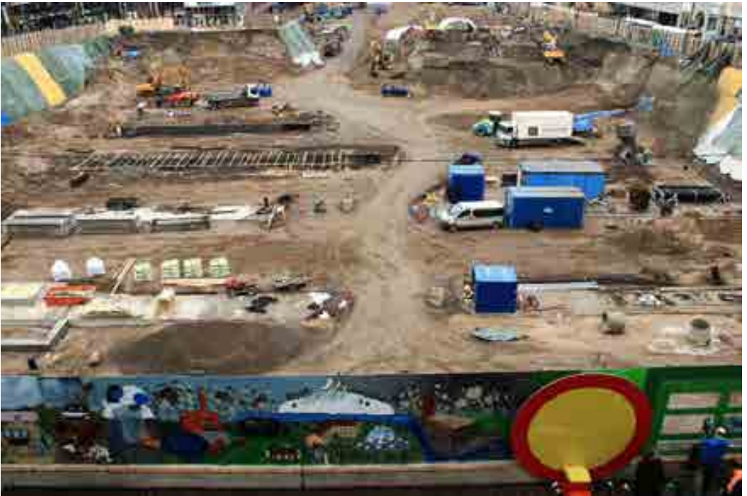
Fig. 6 – The excavation area in the end of the fieldwork period when the final subarea is still unfinished (in the upper right corner of the picture). The whole area was surrounded with a high fence decorated outside with paintings and advertisements. The townspeople were able to follow the work behind the fence through a couple of peepholes covered with plastic (down right in the picture) (Copyright: The Lahti City Museum / Photo library).
