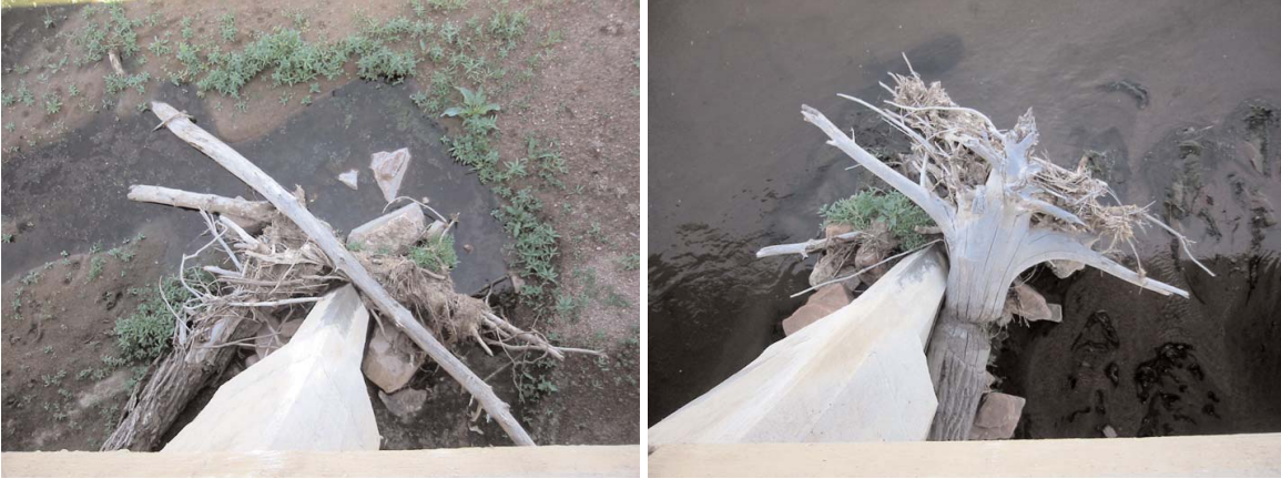
Figure 3-7: debris accumulation at bridge piers (South Platte River, Colorado).
