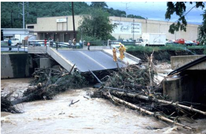
Figure 3-11: bridge failure (NY, USA).
