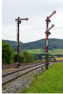
Figure 1.8: A sempahore signal installed along the railway section: source wikipedia
