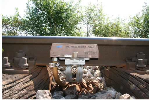
Figure 1.7: An axle counter installed along the railway section: source wikipedia
