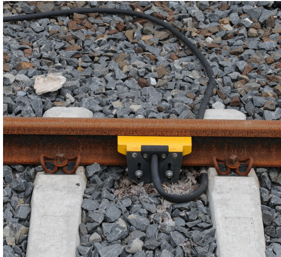
Figure 1.6: A track circuit installed along the railway section: source Wikipedia
