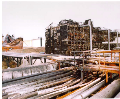
Figure 1.2: Collapse of the piperacks at the Tupras refinery after the Kocaeli earthquake.
