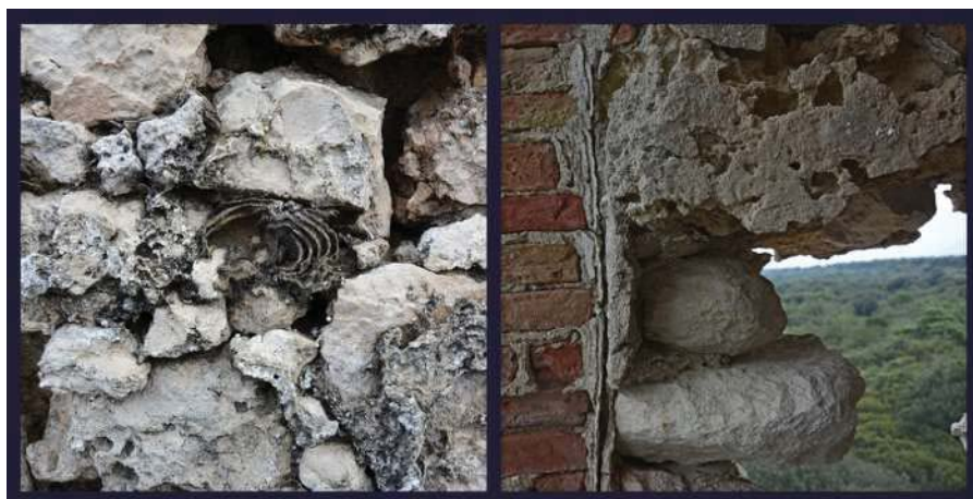
Fig. 04 : Weathering of lime mortars by the marine aerosol
