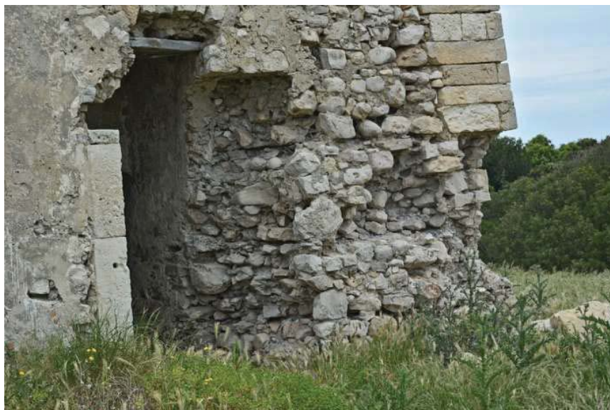
Fig. 03 : Torre Scampamorte. Loss of stone elements from the southern wall
