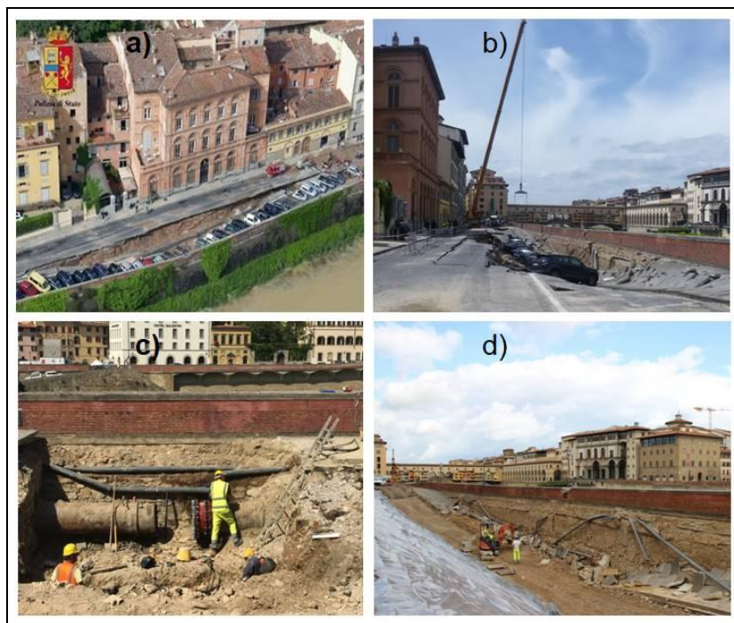
Figure 39. a) Picture from a police helicopter just after the collapse; b) cars removal; c-d) restoration activities.
