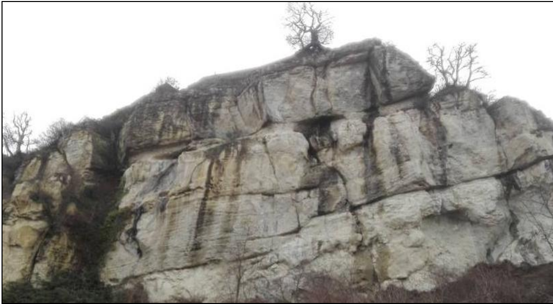
Figure 53. Sub-vertical fractures on the rocky wall of Canossa Cliff.
