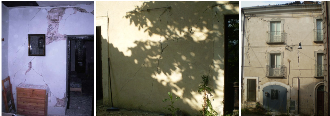
Figure 6-38: Castelnuovo aggregate: diagonal cracking in S.U.4 (left), S.U.6 (centre) and S.U.9 (right).
