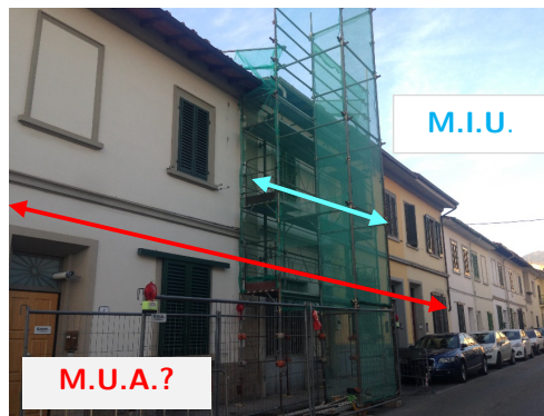
Figure 1-3: M.I.U. in a row aggregate.
