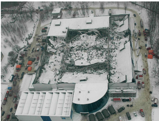
Figure 6.3: Roof collapse Katowice Exhibition Hall.
