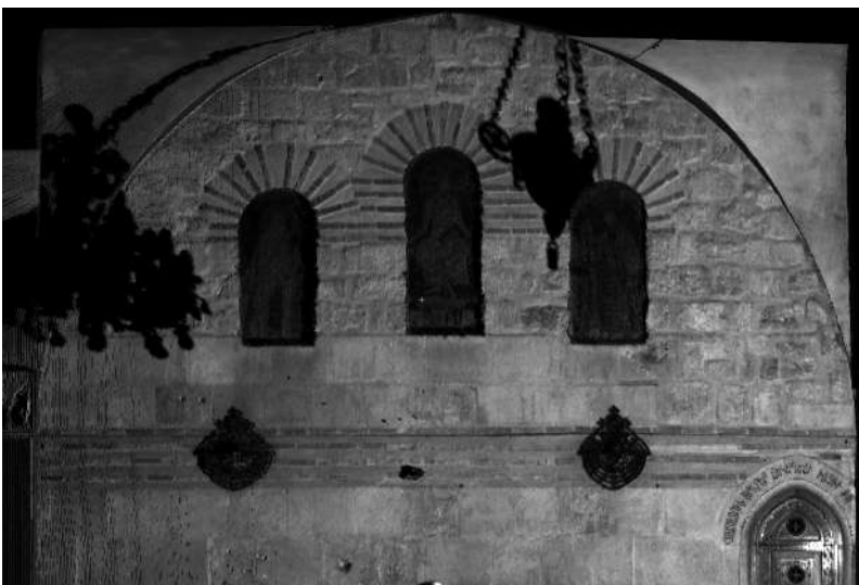
FIGURE 33 South Transept. On the 'point cloud' it is possible to read the typical masonry texture that characterizes the works of Constantine Monomachos.
