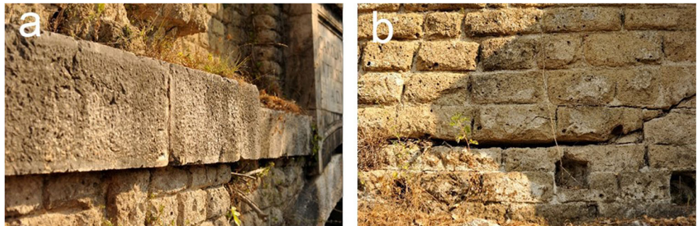
Fig. 4 The main materials of the Bridge: a the local limestone with the presence of a disintegration phenomenon and a superficial patina; b the yellow tuff, and the clear lesion on the South elevation
