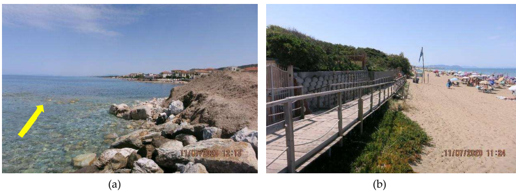
Figure 5-35. Overview respectively from north to south and from south to north of the Subunit A. The yellow arrow in plot a indicates the submerged groin, while in plot b a particular on the upper limit of the active beach is pictured as representative of the upper border within the whole subunit.
