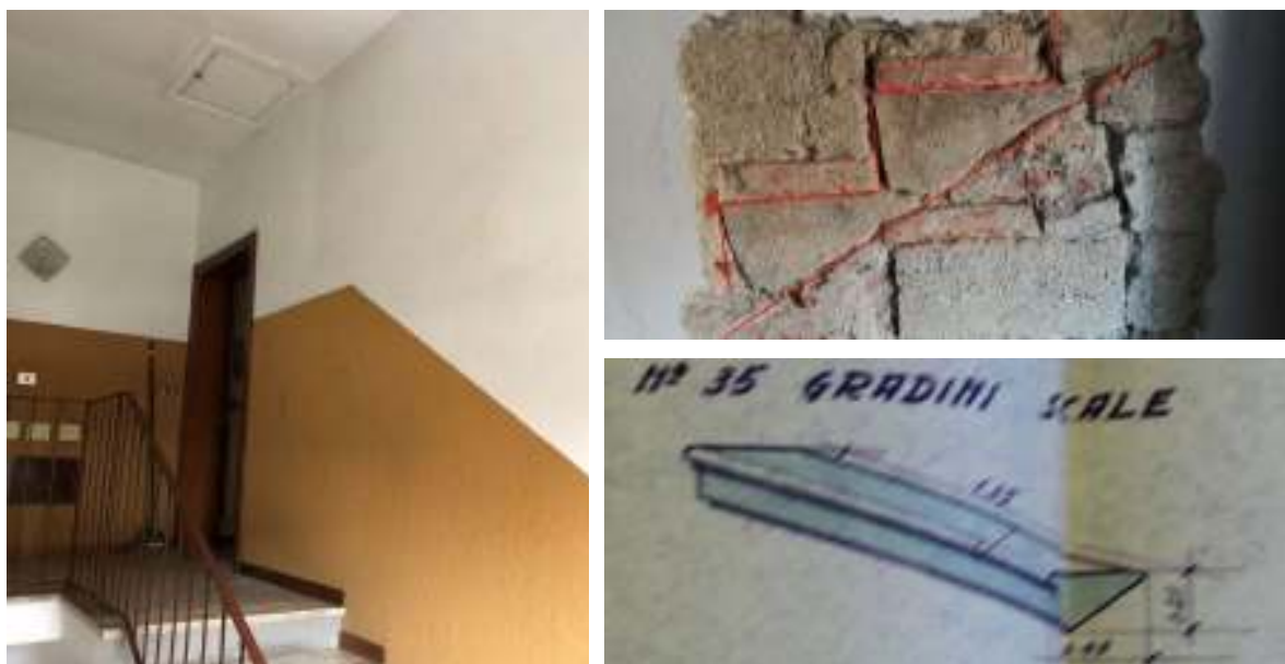
Fig. 2.11. On the left: an internal stair distributing to two apartments for floor. On the right, up: detail of the connection of the steps into the masonry wall; below: drawing of the steps of a stair.
