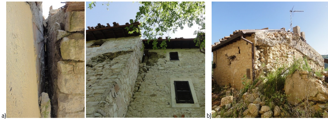
Figure 4.21: Lack of connection between the SUs 142 and 143 (a), as well as among the SUs 151 and 152 (b).
