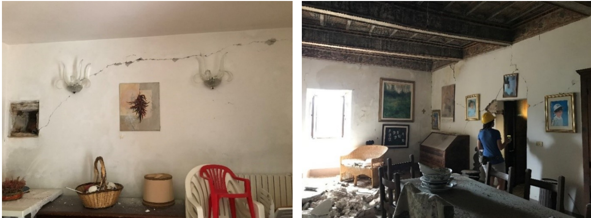
Figure 4.18: Wide cracks in the inner face of the walls inside the SU 117.
