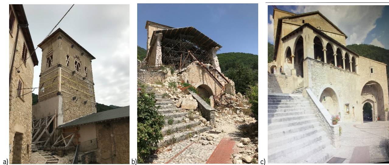
Figure 4.8: Saint Andrea Church Tower secured after the 2016 earthquake (a), façade of the Church and medieval gate of the town after seismic event (b) and before (c).
