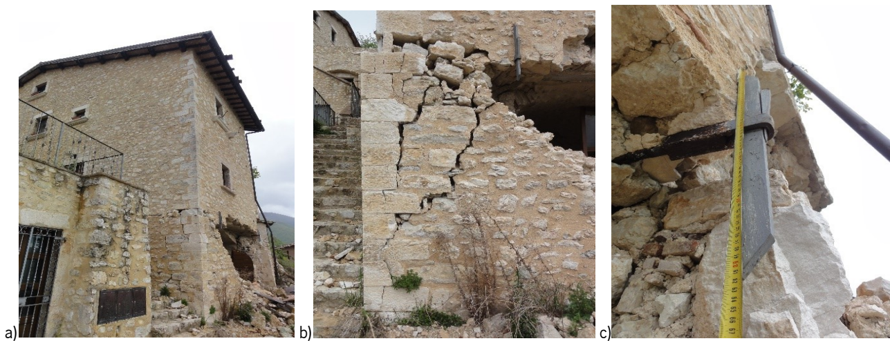
Figure 6.11: Overturning of the wall of the ground floor (SU 112) (a) and detail of the tie of the façade (SU 112) (b, c).
