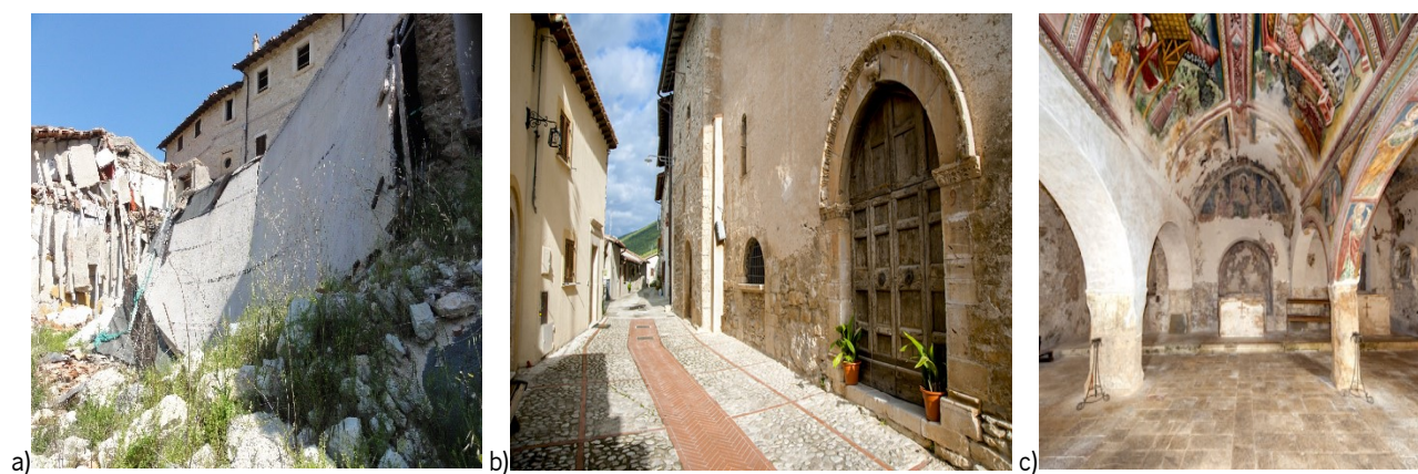
Figure 4.10: Saint Maria di Piazza church after the earthquake 2016 (a) and before outside (b) and inside.
