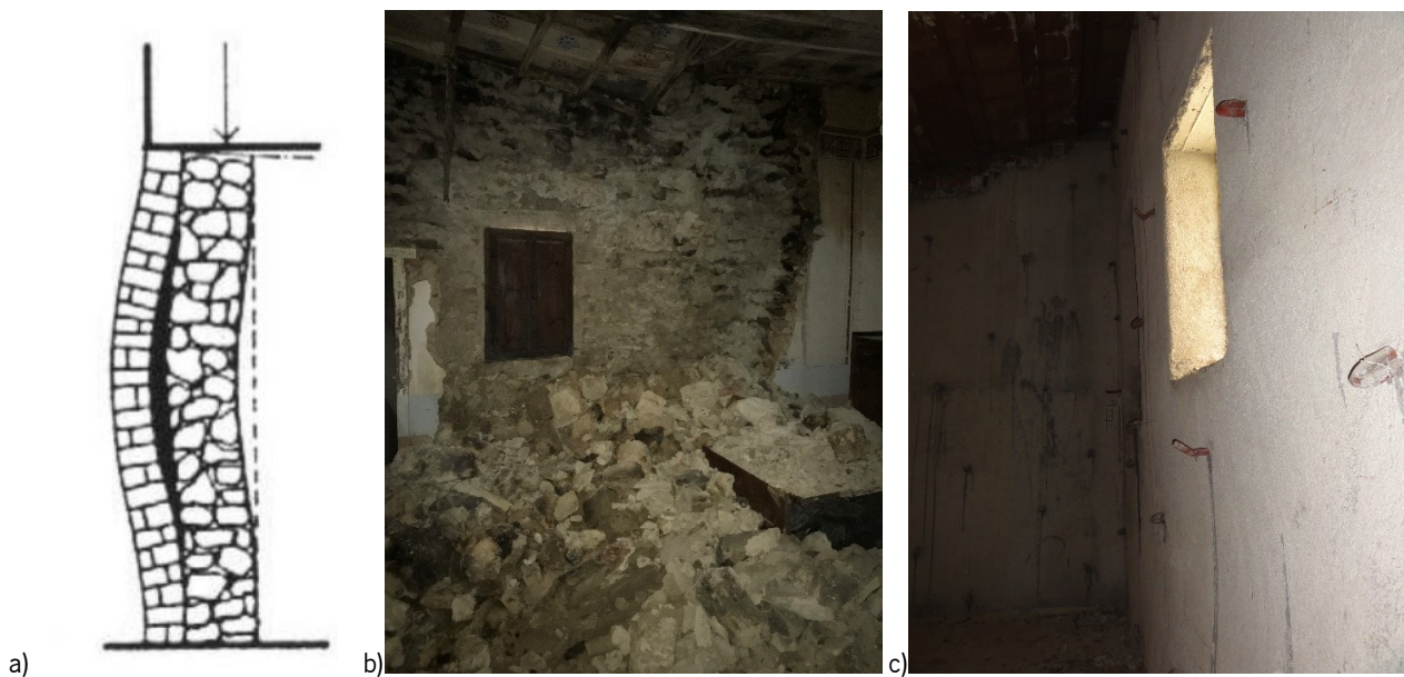
Figure 4.24: Scheme of the failure mechanism due to masonry instability (a); Internal photo of SU 117.2, where the absence of transverse connections of the double leaves of the wall didn't allow the development of flexural/shear behaviour and the collapse occurred due to instability of the internal wall panel (b); The previous image is compared with the one collected in SU 168, in which an old retrofit technique, consisting of using the reinforced concrete with welded mesh and mortar injections, prevented an instability collapse.
