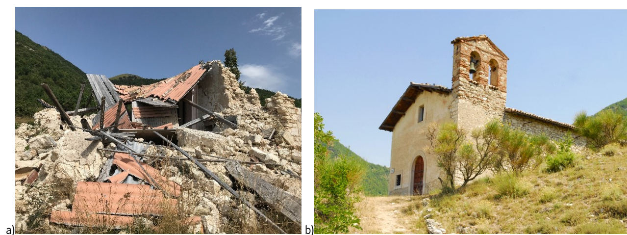
Figure 4.9: Madonna della Neve church after the earthquake 2016 (a) and before (b).
