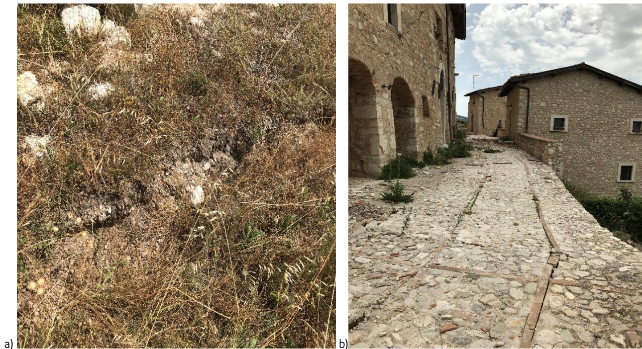
Figure 4.7: Ground crack detected under the dense vegetation (a) and street collapse of Via del Cucolo due to the overturning mechanism of the retaining wall (b).
