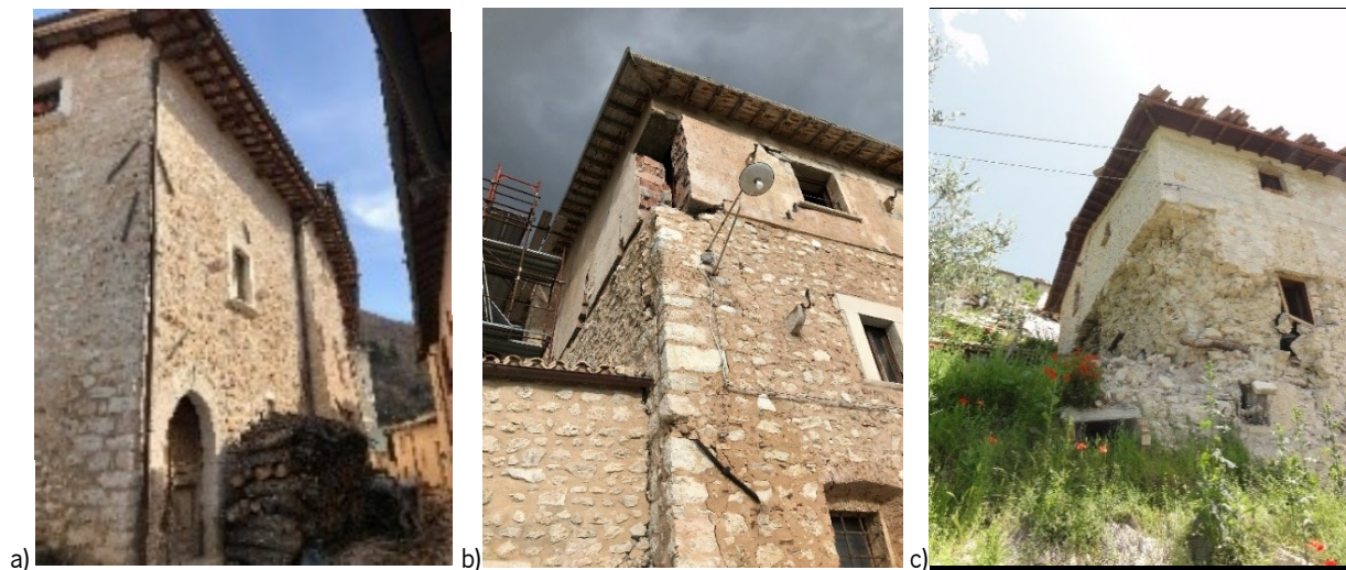
Figure 6.13: Presence of tie rods at the corner of the aggregate (SU196) (a); Corner failure of external buildings of an aggregate, caused by the absence of tie rods (SU 60) (b) and masonry connection between two orthogonal walls (SU 142) (c);
