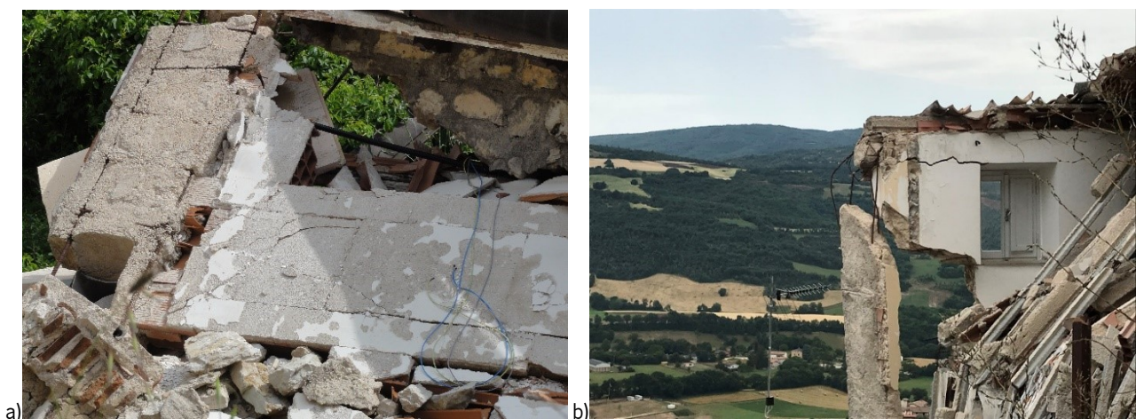
Figure 4. 22: Inferior part of a reinforced concrete ring without elements (steel bars, glass fibers) that guarantee the connection with the masonry detected in the SU 155 (a); Portion of reinforced concrete ring, hanging from the roof of SU 183 (b).
