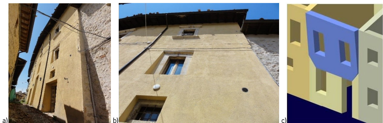
Figure C. 9: Activation of the partial overturning of the façade, a mechanism that is characterised by a horizontal crack in the final part of the buttress.
