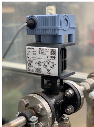
Figure 65. The 3-way valve mounted in cold circuit.
