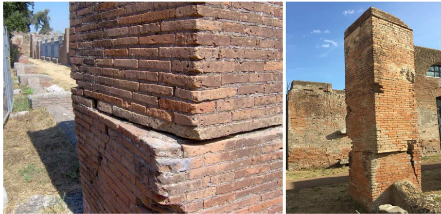
Fig. 6. Historic damage in one of the pillars of the “Piccolo Mercato”. The fracture zone due to the twisting of the pillar is clearly visible.
