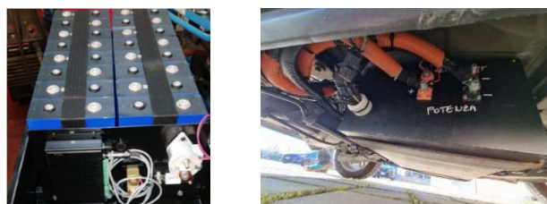
Fig. 6. Installatio of the Battery under the Smart Prototype
