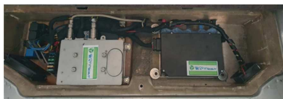
Fig. 7. Installatio of powe electronics on the Smart Prototype (motor controller and battery AC/DC rectifier)
