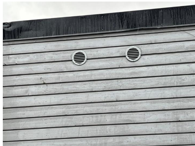
Figure 3.20: Openings made in the technical cabin to exchange heat with the surrounding air.
