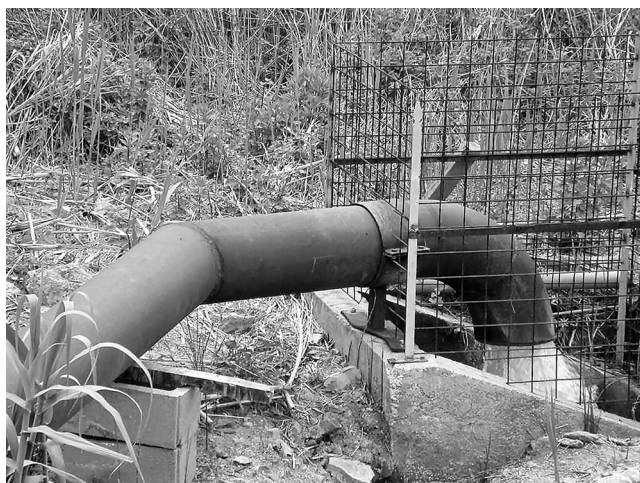
Figure 15. Water pumping system at the Gavorrano underground mine (at present, about 80 L/s)
