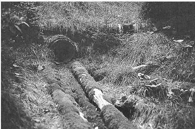
Figure 7. Water outlet before water outburst in 1998
