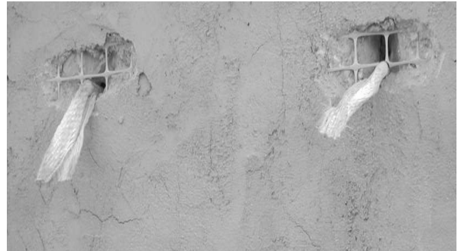
Figure 8 Connection between through anchors and polypropylene reinforcement: bars are wrapped with GFRP sheets and fixed to the polypropylene mesh using epoxy-resins
