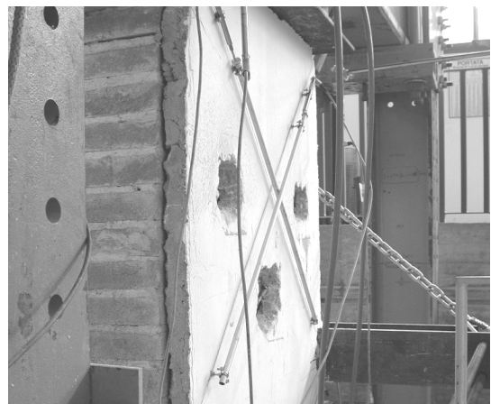
Figure 16 Ferro-cement: failure mechanism
