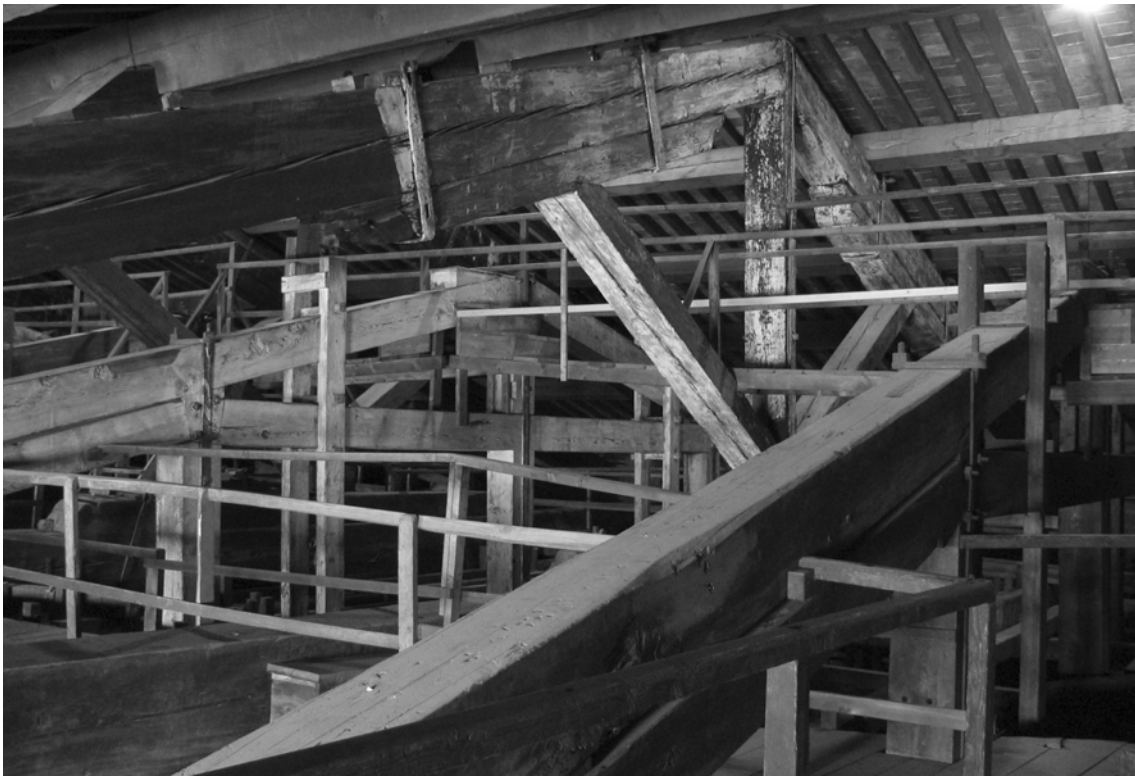
Figure 2: Panoramic view of the “Salone dei 500” garret, in the middle the vasarian trusses.
