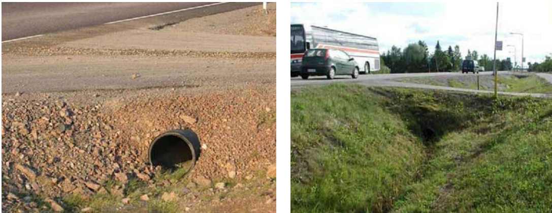
Figure 11: Examples for hazardous drainage features (Source: [A.2])
