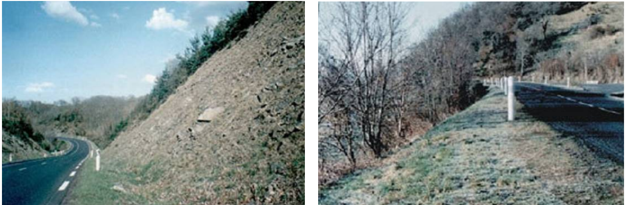
Figure 12: Examples for hazardous cut (left) and fill slopes (right) (Source: [A.2])
