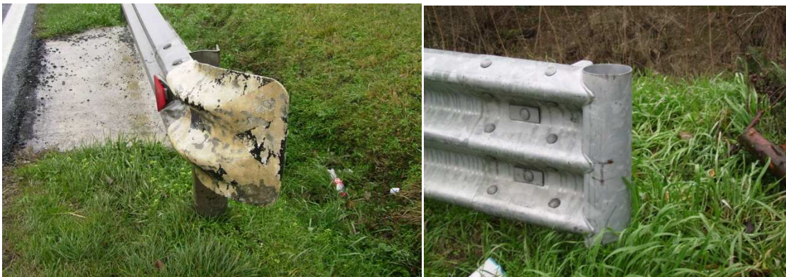
Figure 2: Unprotected (or “exposed”) terminals
