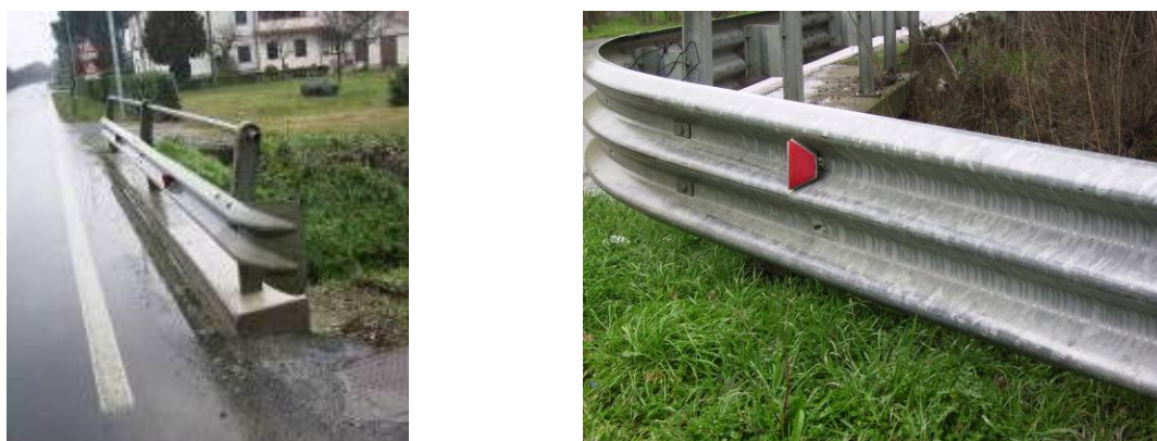
Figure 9. Type "a" barrier terminal (left) and barrier curved in the driveway that is not considered as un "unprotected" terminal (right).
