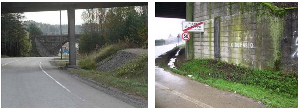
Figure 8: Examples for a hazardous bridge abutment (left) and overpass (right) (Source: [A.2])
