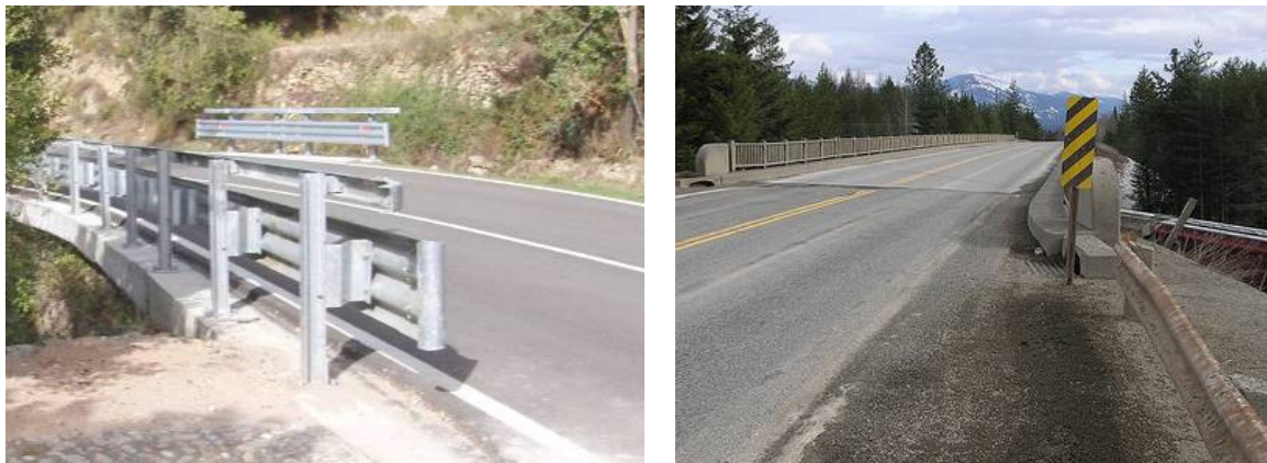
Figure 9: Examples for hazardous safety barrier terminations
