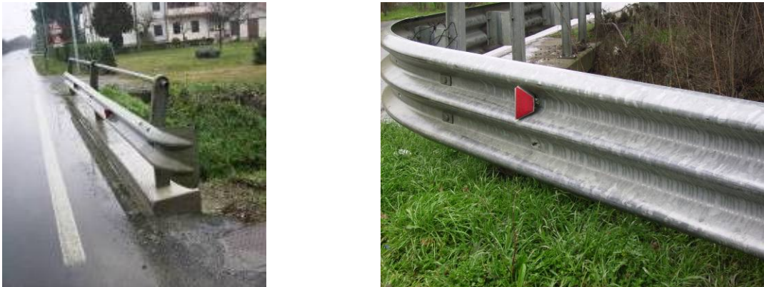
Figure 9. Type "a" barrier terminal (left) and barrier curved in the driveway that is not considered as un "unprotected" terminal (right).
