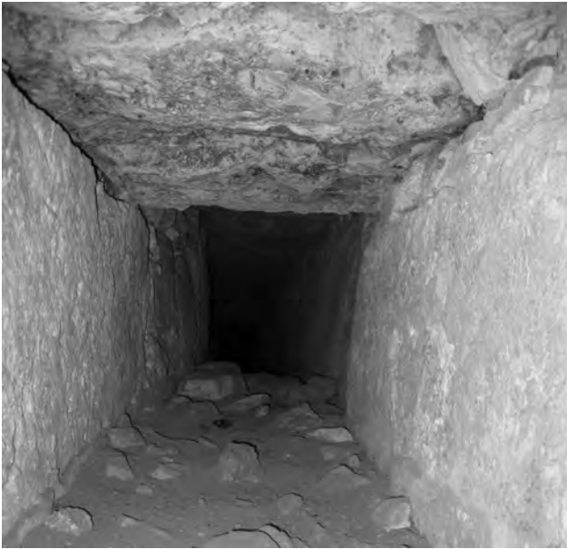
Fig 17 - Guest house: ground floor, pipe in the rock wall of the first room.
