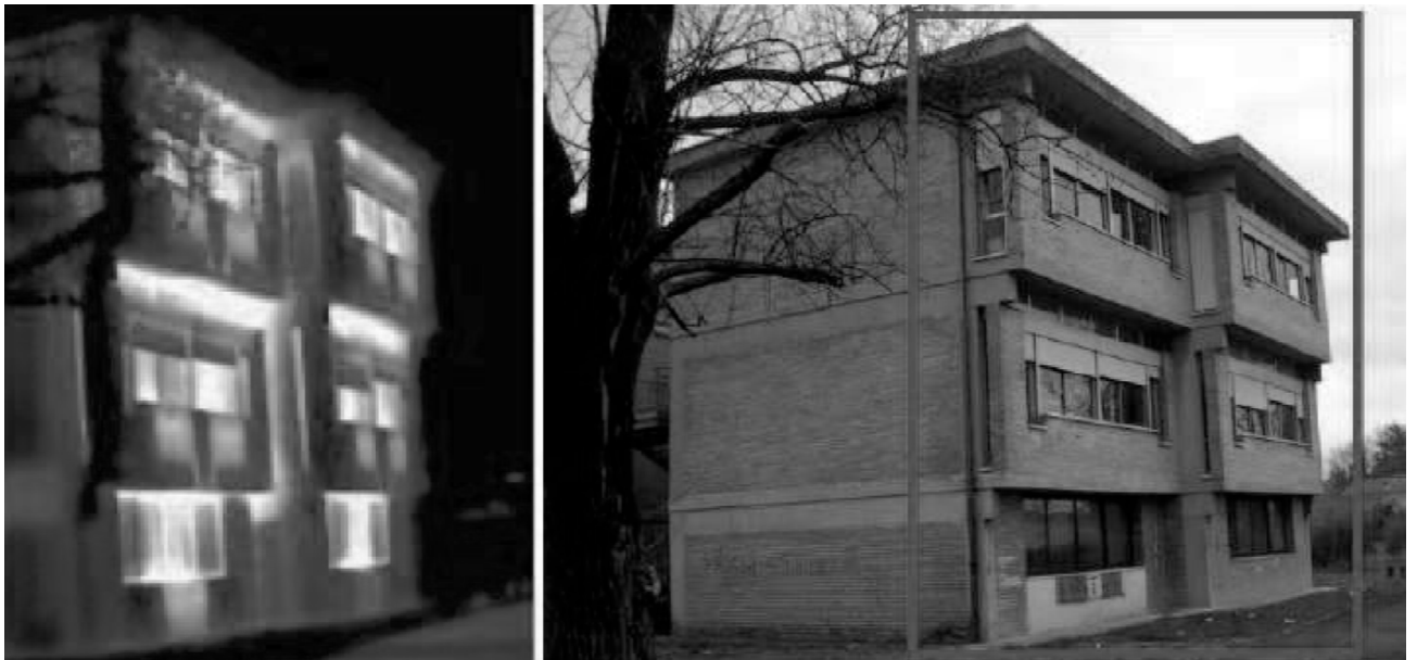
Figure1: Thermography has been a fundamental instrument in the diagnosis phase: heat losses can be localized easily
