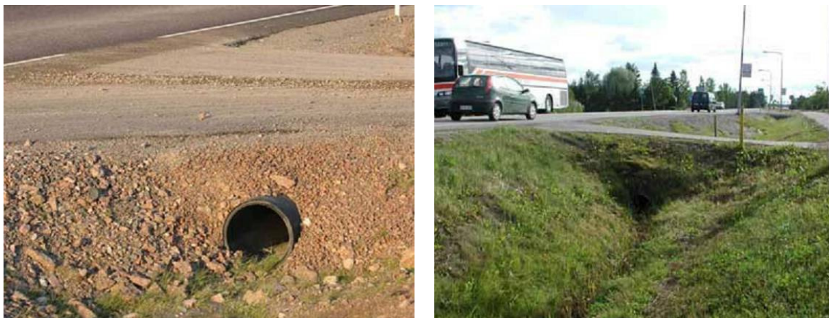
Figure 55: Examples of hazardous drainage features (Source: [A.2])
