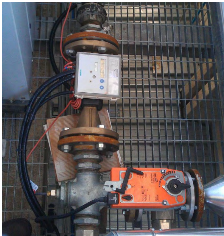
Figure 54 - Energy meter of the electric chiller
