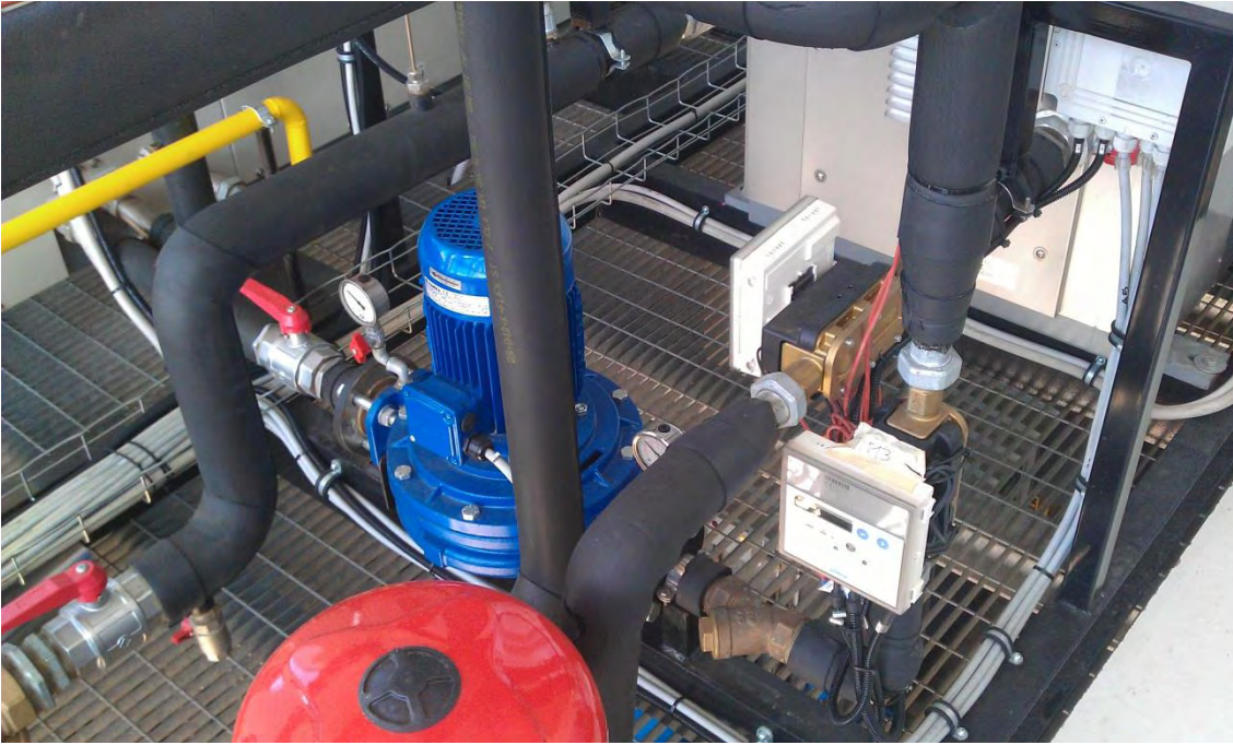
Figure 53 - Energy meters of the CHP (left) and the absorption chiller (right)
