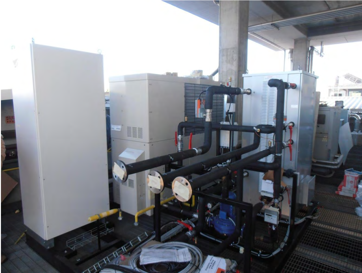
Figure 27 - Skid of the tri-generation system
