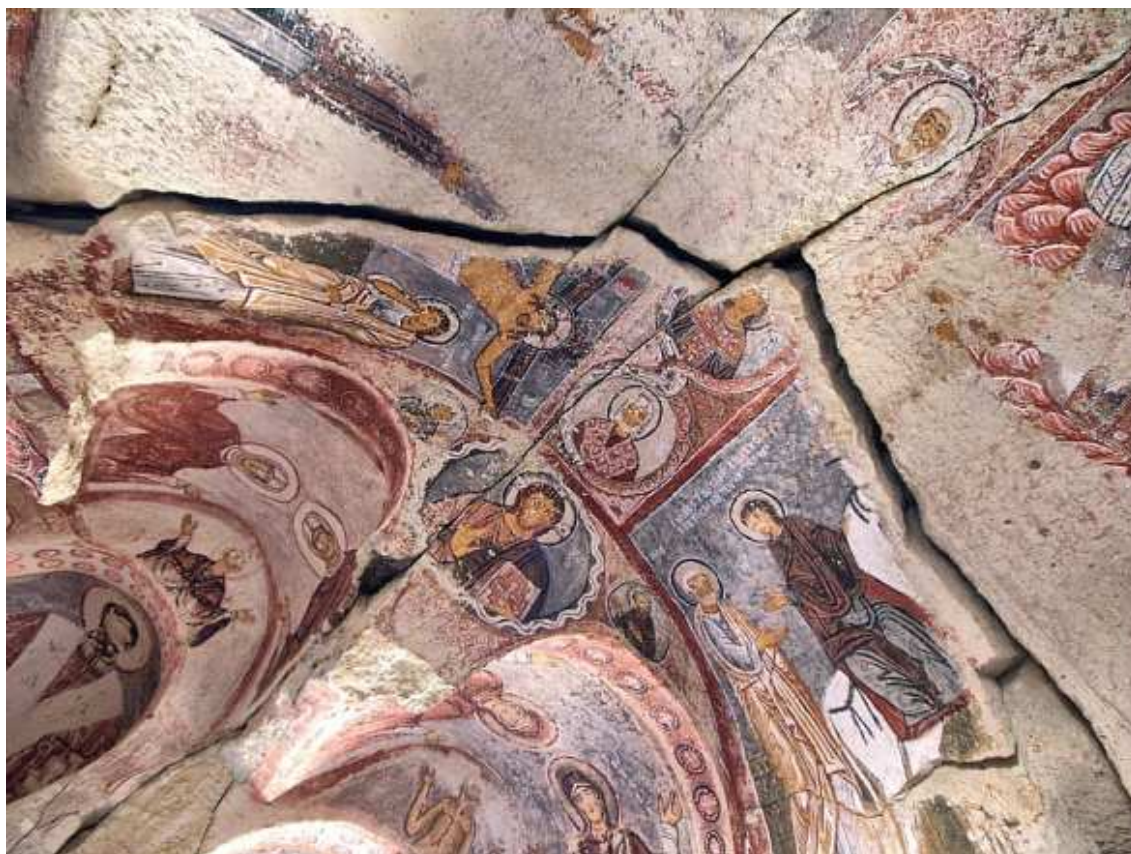
Fig. 2 – The great crack passing all over the vaults
