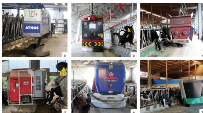
Fig. 1 Different models of AFS: a) rail-suspended only distributor; b) Wheel-driven; c) rail-suspended chopper-mixing and distributor; d, e, f) Self-propelled (pictures taken by the authors)
