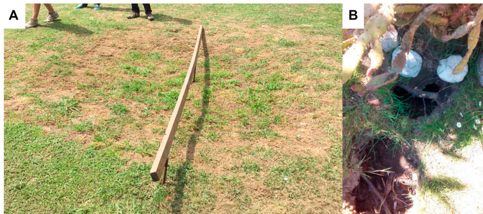
FIGURE 3 (A) localized subsidence spotted in 2015, 300 m from the 1995 event (see Figure 4 ); (B) small cavities occurred in Camaiore.
