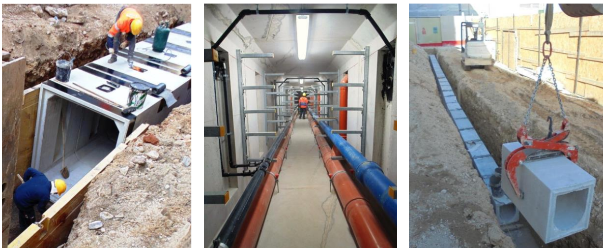
Figure 1. The Smart Tunnel under construction (left); view from inside the tunnel, with installed wastewater and water supply pipes (center); the top channel for the collection of rainwater (right).
