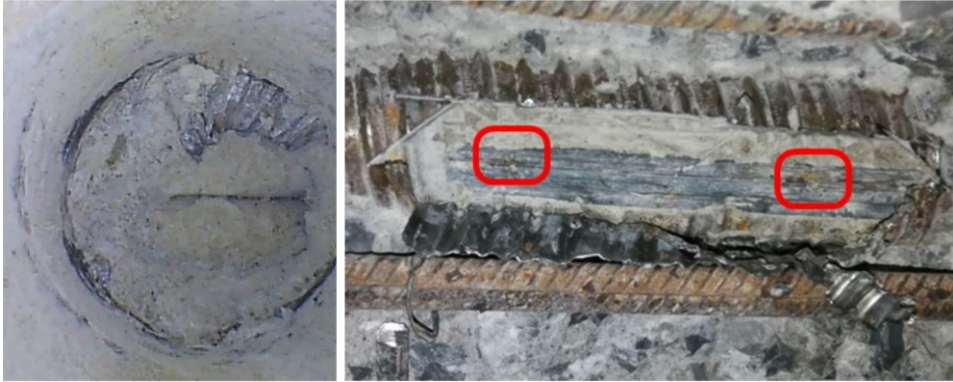
Figure 5-7: Data from the inspection campaign. Left: an endoscopic inspection showing a fully grouted and uncorroded cable. Right: a destructive inspection revealing wire corrosion (circled in red) despite the duct being fully grouted.
