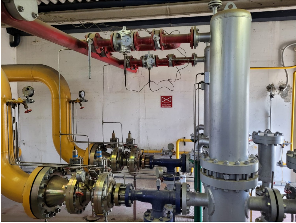
Figure 1.10: CGS preheating heat exchangers and monitors for pressure reduction stage.
