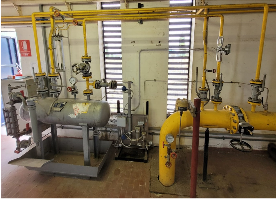
Figure 1.12: CGS odorization stage: injection and lapping systems in series.
