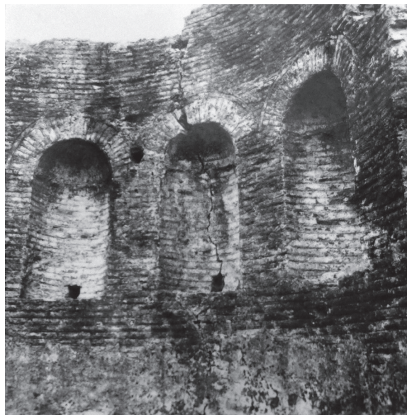
294. East wall of the Nymphaeum after the paint restorations: between the north and the central niche, the presence of a circular hole for a post of the iconostasis of the medieval church.
