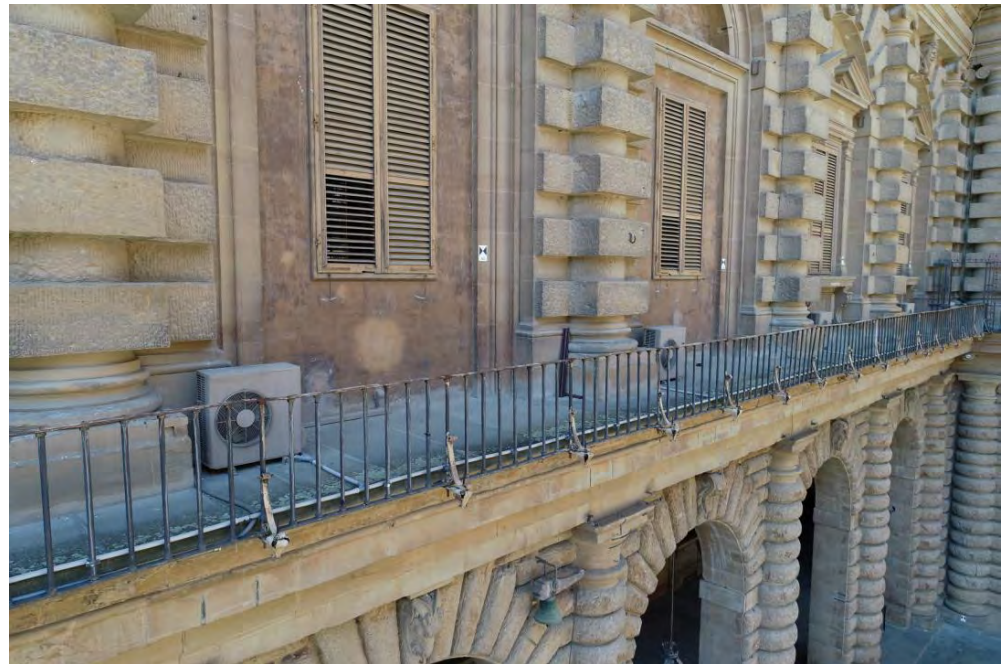
Figure 19. Air conditioning systems on the terrace of the second floor. Such elements can be wrongly classified.
