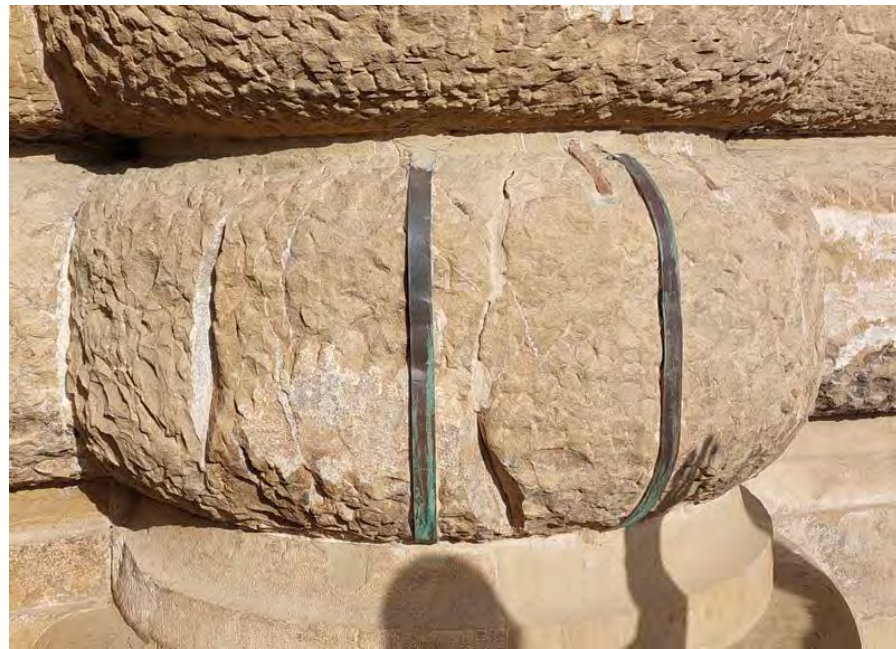
Figure 4. An example of a broken ashlar fixed with several types of metal ties over time.
