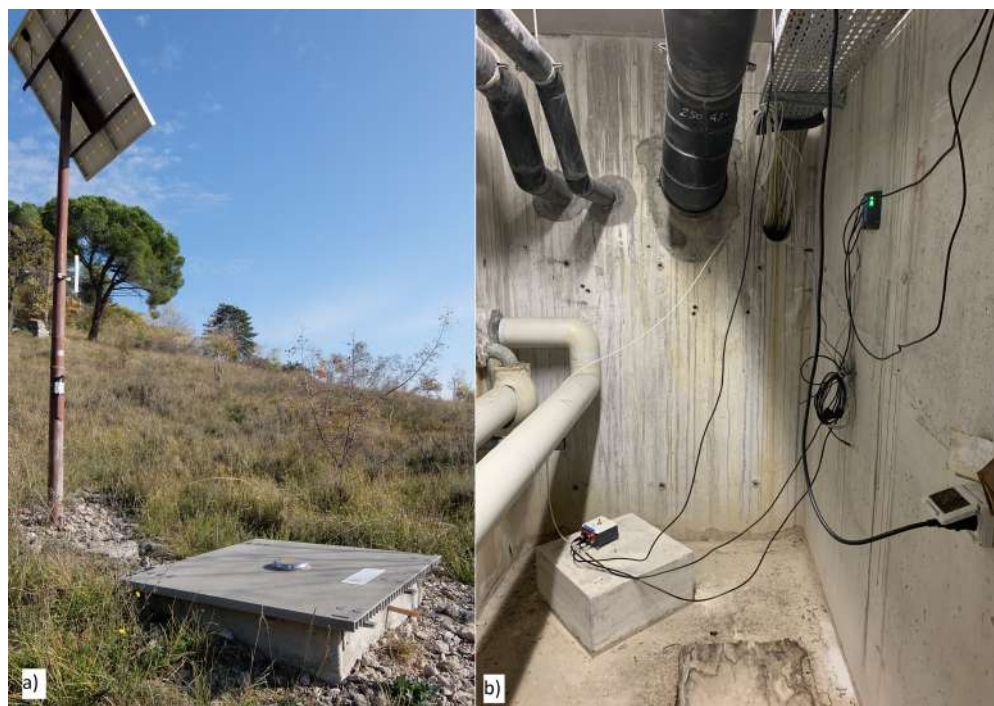
Figure 2. The two typical (a) free-field and (b) inside-buildings installations used in the RAN network. (a) is the the MONF station, while (b) is the POR one.
