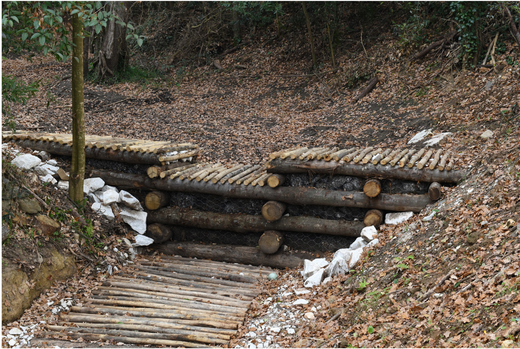
Fig. 2. Wooden check dam at the outlet of Santo Pietro watershed (photo by P. Trucchi).
