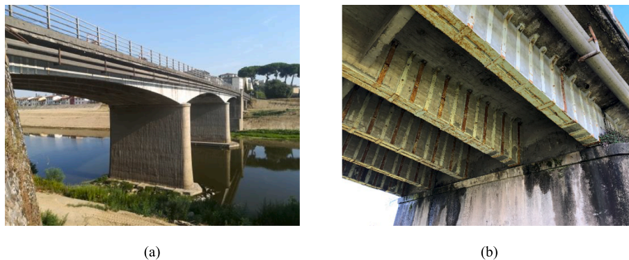
Fig. 1. Views of the Ponte Nuovo bridge: (a) from the Lastra a Signa, side and (b) details of the strengthening steel bars (beton plaqu  technique) installed in the past.
