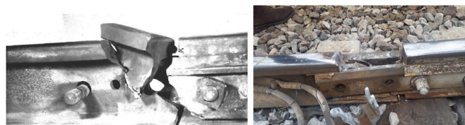
Fig. 3. Broken IRJ in Hither Green, UK (1967) and in Piolotello, Italy (2018). (For interpretation of the references to colour in this figure legend, the reader is referred to the Web version of this article.)
