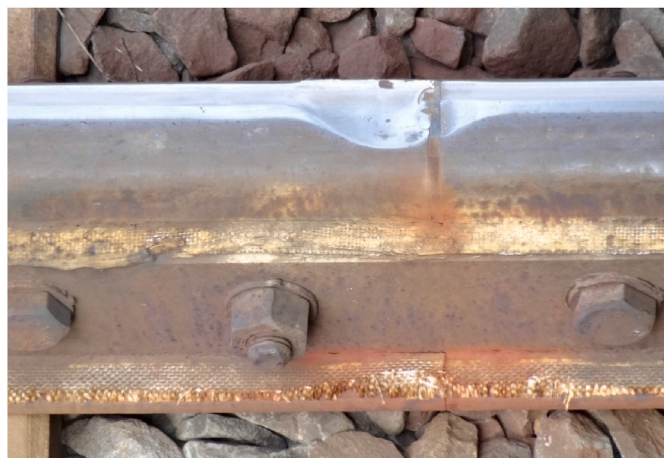
Fig. 1. IRJ with heavy plastic deformation generated by dynamic forces at each wheel passage. Insulating elements are clearly damaged (Photo by the authors).
