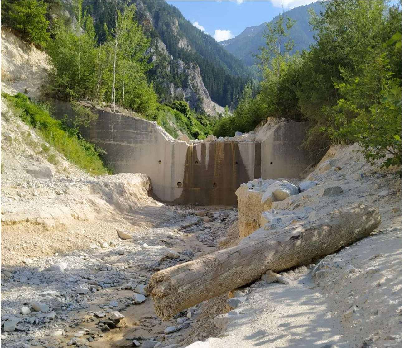
Figure 1. 15: photo of the Check Dam 20, one of the 30 check dams built in the Illgraben channel at the end of the '60s. The dam is ~8 m high (source: Giacomo Belli).
