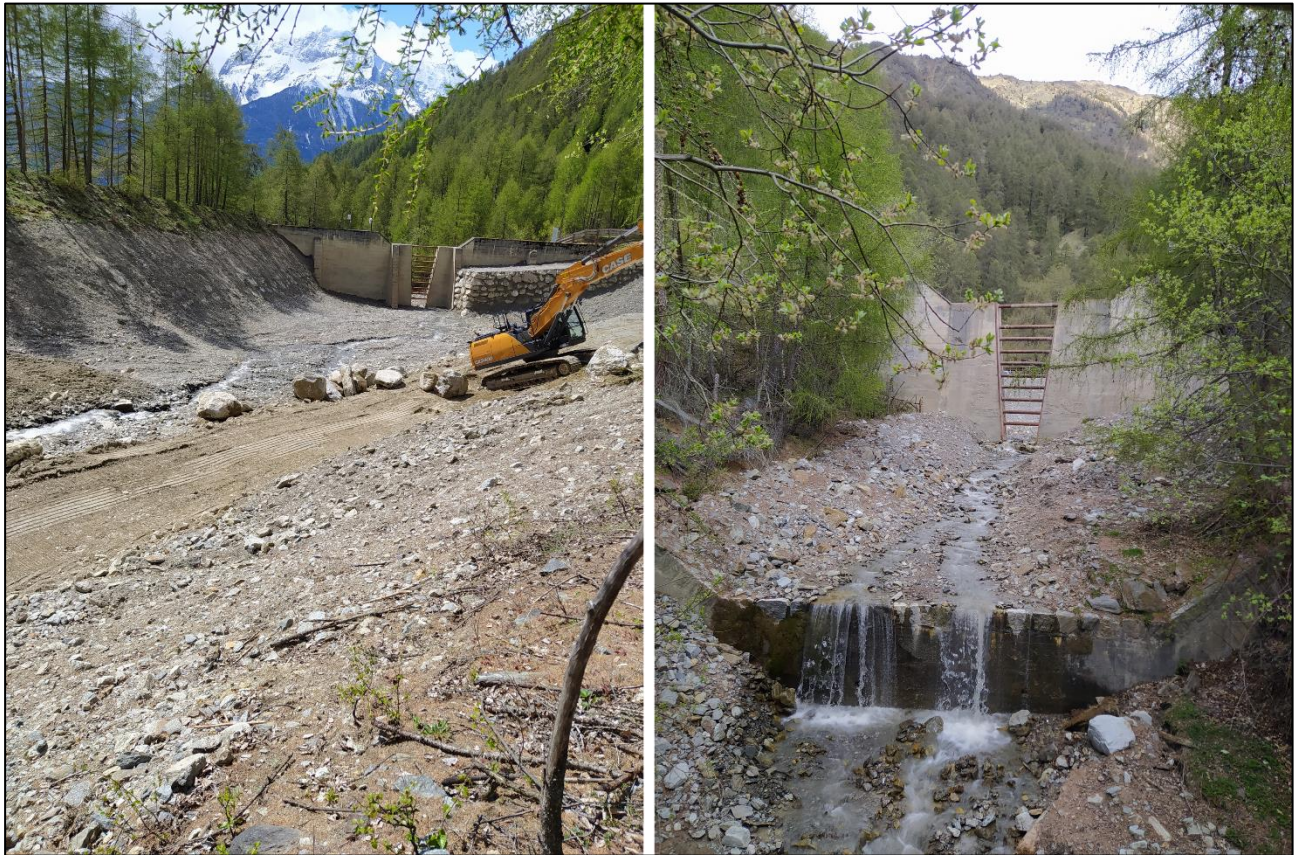
Figure 1. 17: upstream (left) and downstream (right) sides of the ~10 m high filter check dam built in the Gatria basin in the '70s (source: Giacomo Belli).
