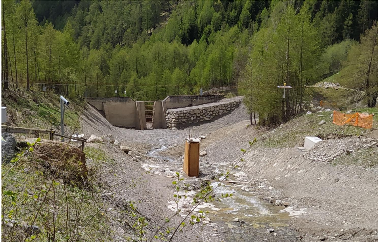
Figure 1. 22: photo showing different sensors and devices installed in the Gatria channel (Bolzano, Italy) for debris-flow study, monitoring and risk reduction, including the filter check dam in the background, the sensor pillar for flow impact measurements in the middle of the channel, an altimeter suspended over the channel and a camera on the left bank (source: Giacomo Belli).
