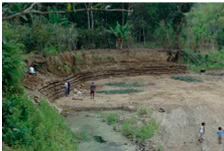
Figure 2. Water bioengineering (WBE) construction at Las Maravillas after the finalization in 2008 (Petrone, 2008).
