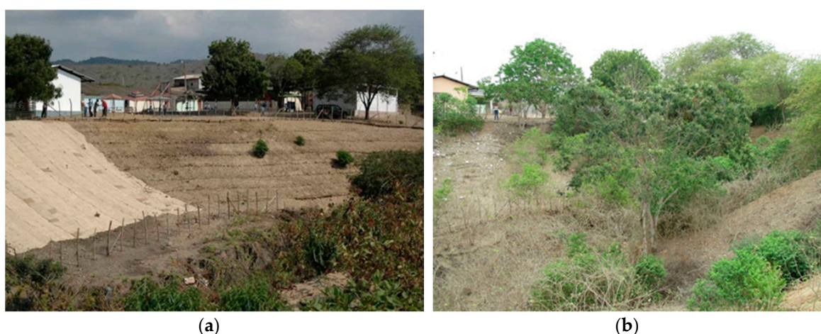
Figure 10. SBE construction at Membrillar (a) after the finalization in 2008 (Petroni, 2008); (b) monitoring in 2018 (Maxwald, 2018).
