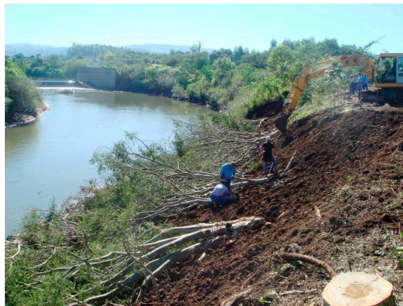
Figure 8. WBE construction at Santa Cruz do Sul after the finalization in 2010 (Suttili F.J., 2010).
