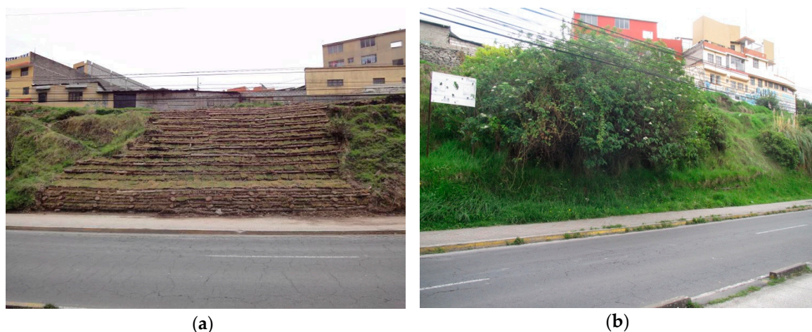
Figure 4. SBE construction at Av. Maldonado in Quito (a) after the finalization in 2012 (Petrone, 2012); (b) monitoring in 2018 (Maxwald, 2018).
