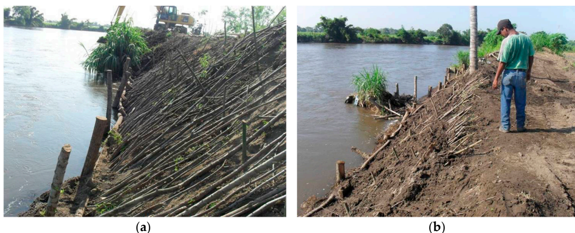
Figure 3. WBE construction at La Nueva Concepción (a) single walled crib wall at the base and living branches at the slope (Petrone, 2009); (b) after the finalization in 2009 (Petrone, 2009).
