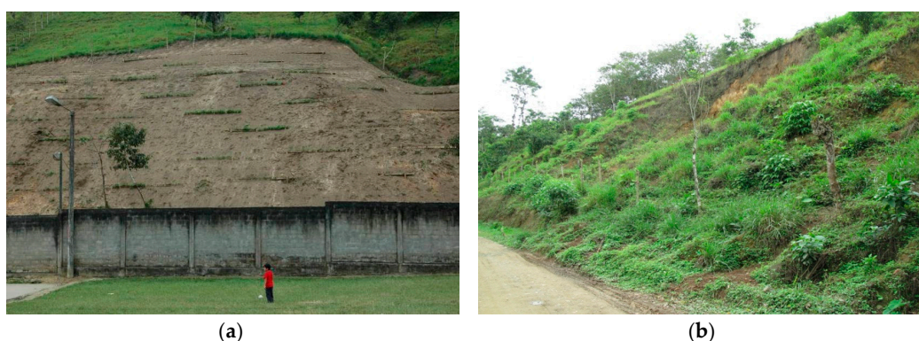
Figure 11. SBE construction at San Miguél (a) after the finalization in 2010 (Petroni, 2010); (b) monitoring in 2018 (Maxwald, 2018).
