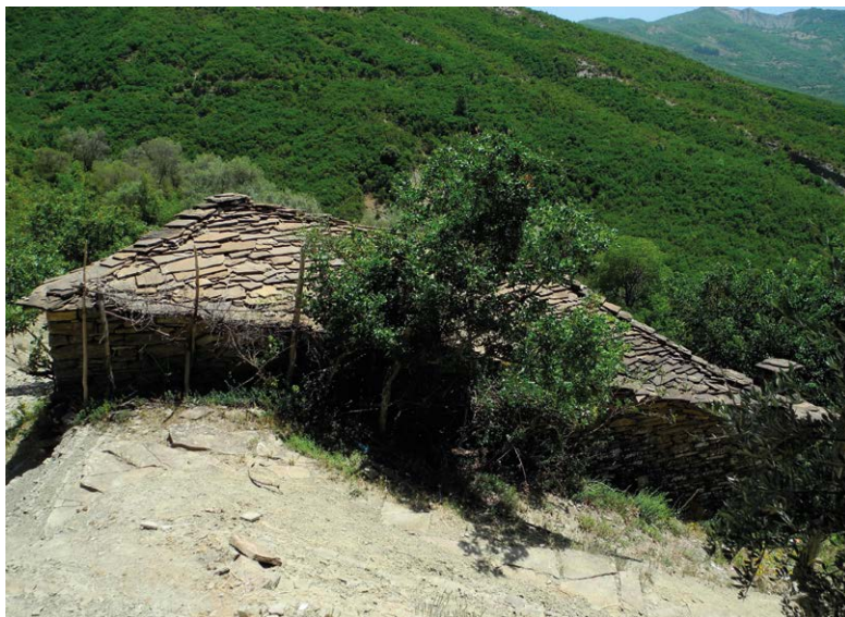
Figure 3.33 – Roofing of a building made of the same slabstone used for the path.
