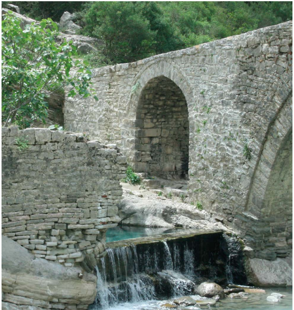
Figure 3.37 – Abutment of the Kadiu Bridge and thermal pool, detail of the archway springer and the side archway.
