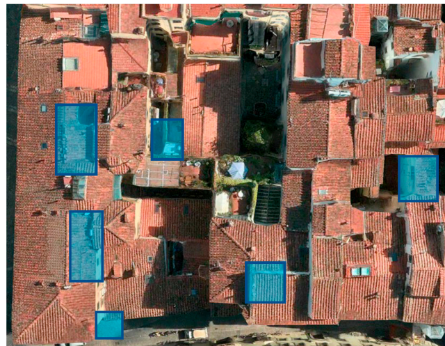
Figure 5. An example of the prospect and roof degradation recognition—blue area: differential degradation.
