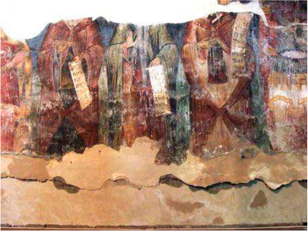
Figure I-5.3.11 Severe damage on the south wall of the church due to the rising damp.
