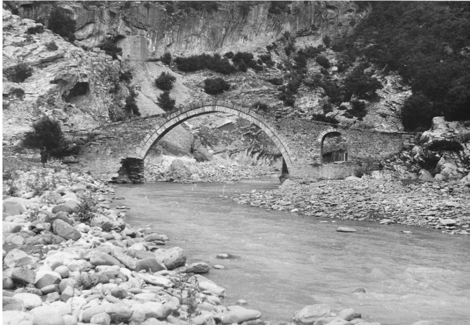
Figure I-5.1.1 View of the Katiu Bridge before the restoration works in 1982 showing the damage suffered by the left abutment (looking upstream) during World War II. [Courtesy: Municipality of Përmet]
