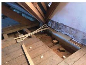
Figure 8 – Repair of connections between roof structure with floor beams (credits: Aníbal Costa)
