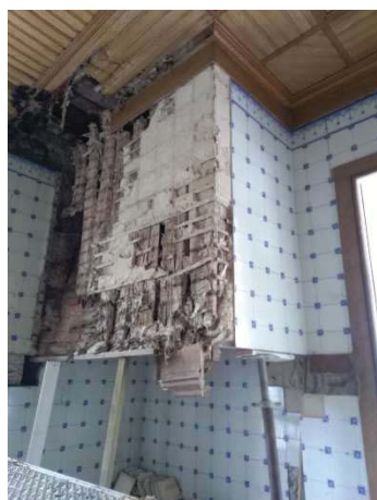
Figure 4 – Leaks through the roof, chimney, kitchen (credits: Aníbal Costa)
