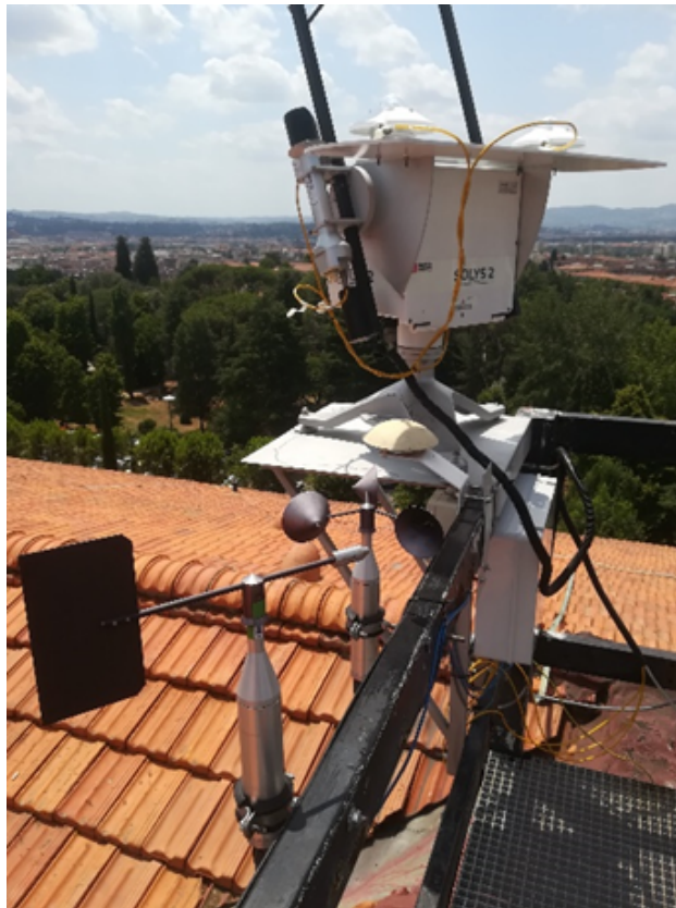
Figure 5.8: Weather station over the roof of Santa Marta Engineering faculty in Florence
