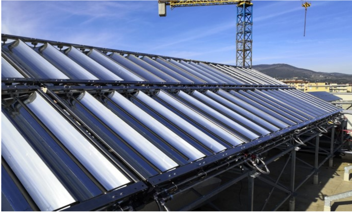
Figure 2.14: m-PTC field of Torre degli Agli pilot project
