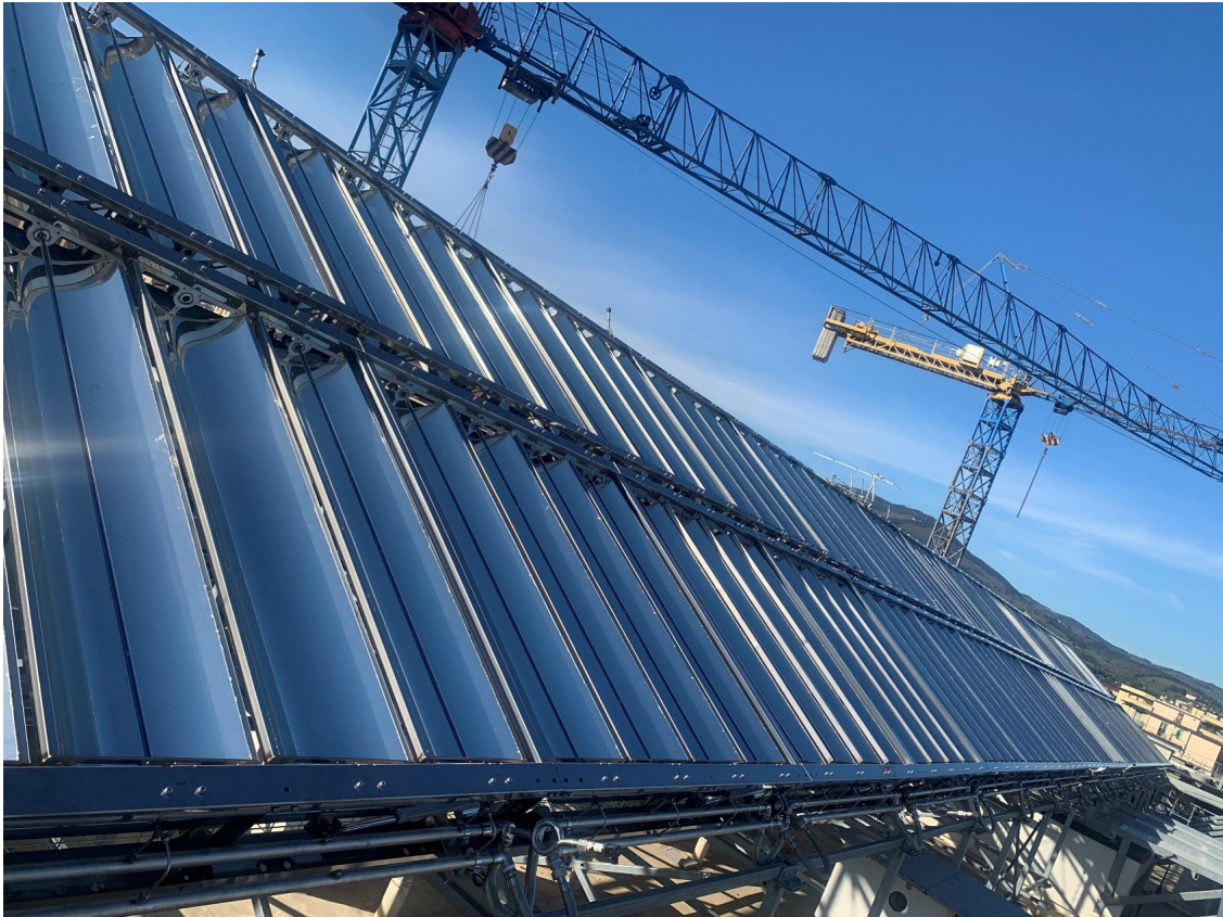
Figure 2.12: m-PTC field of Torre degli Agli pilot project
