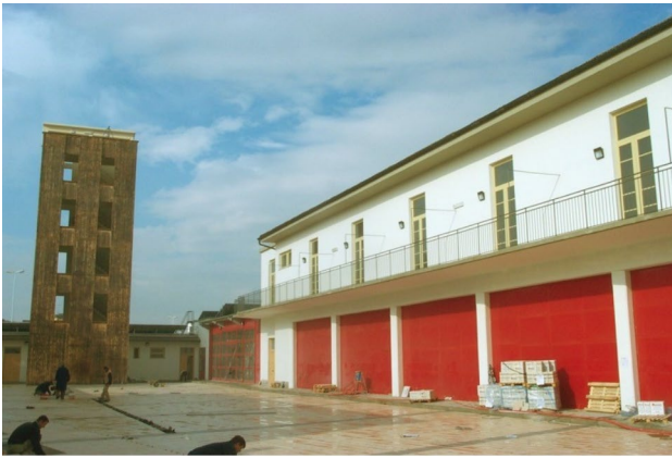
Fig. 1 Side view of the former firehouse in Prato during the renovation works
