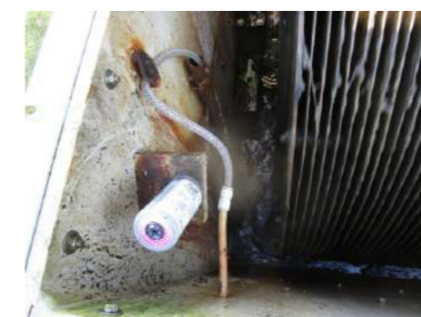
Figure 2. Injection of iron chloride inside the biological rotating disc tank.
