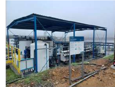
Figure 1. LIFE REMINE WATER pilot plant.
