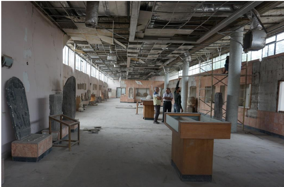
Fig. 5. June 2023. Post-earthquake damage assessment on the first floor of the museum building with ReStruere and Unifi team. guests ©Aleppo project
