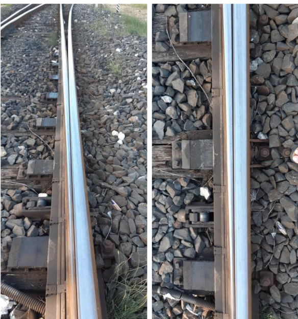
Figure 20. Closed switch rail / stock rail pair of an old and heavily loaded turnout. The load transfer is smooth and no damages are visible
