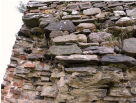
Fig. 6- The small, roughly hewn ashlars of grey to green-purple quartzite constituting most part of the perimeter walls (photo by Fabio Fratini, 2022)
