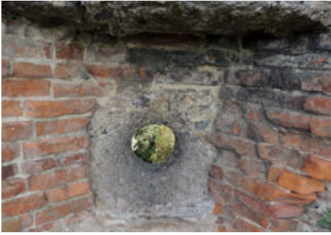
Fig. 4- A fire mouth with the hole and lintel made of Verrucano conglomerate (photo by Fabio Fratini, 2022)
